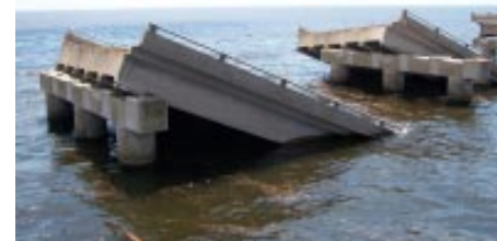
I-10 over Lake Pontchartrain, Orleans Parish, Louisiana. The concrete bridge was built as a series of simply supported prestressed spans, prefabricated off-site for ease of construction.
